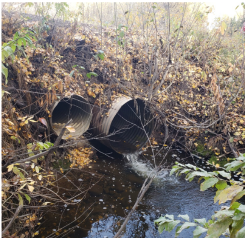
Photo 1. Perched culverts at Dog Creek FSR.
